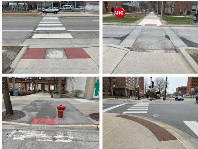
Figures | Top: (Left) Detectable warning strip partially missing at Damen Avenue near the VA; (Right) Detectable warning strip is altogether missing at the inner drive east of Damen Avenue across from the VA; Bottom: (Left) Detectable warning strip on Paulina Street; (Right) Elongated detectable warning strip at Damen Avenue and Polk Street
