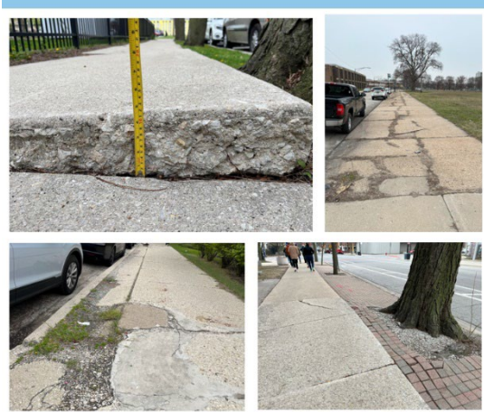
Figures | Top: (Left) Uneven sidewalk, over 4 inches, on Campbell Park Drive; (Right) Sidewalk on Seeley Avenue in poor condition; Bottom: (Left) Crumbled sidewalk on Taylor Street; (Right) Uneven sidewalk on Polk Street
